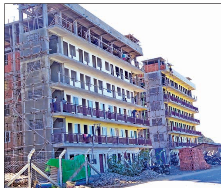
Six storey buildings under construction for renting them to low-income people. PHOTO: MAUNG PYI THU
