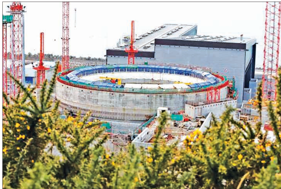
General view of the construction site of the third-generation European Pressurised Water nuclear reactor (EPR) in Flamanville, north-western France in 2013. PHOTO: REUTERS
