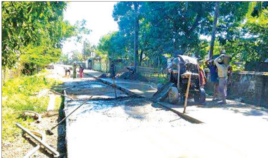
Reinforced concrete road under construction in Ngathaingyoung. PHOTO: SOE MIN OO (IPRD)
