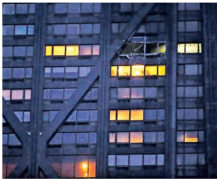
Windows are seen missing from the 50 th floor of the John Hancock Centre after a 2-11 alarm fire was extinguished by firefighters in Chicago, Illinois on 21 November. PHOTO: REUTERS
