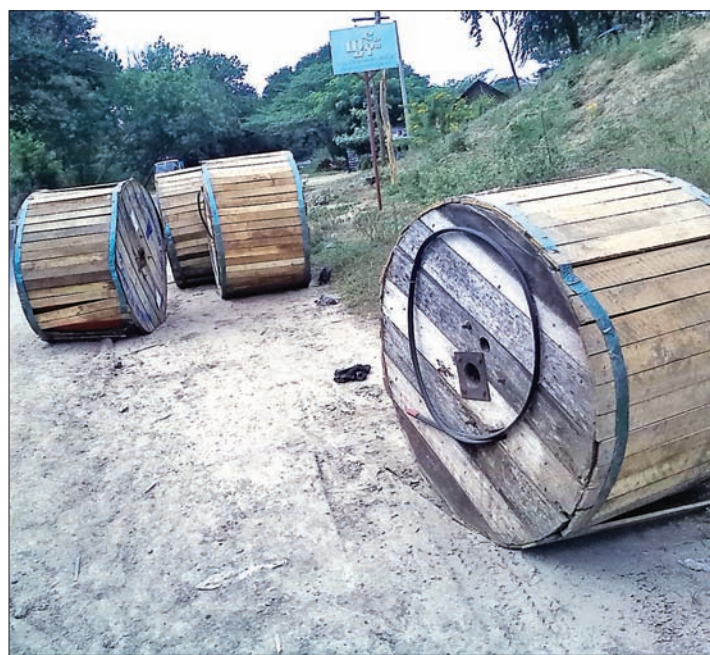
MPT starts installation of cables in Natogyi Township to create GSM access to local people. PHOTO: HTAY MYINT MAUNG
