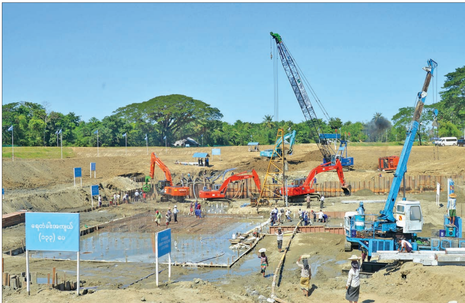
Engineers and skilled workers building Mezali sluice gate (2) in Nyaungdon Township. PHOTO: MNA
