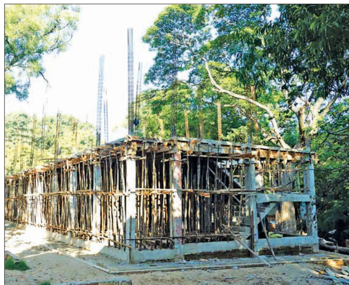
A school building under construction for basic education school in Meiktila District. PHOTO: CHANTHA -MEIKTILA
