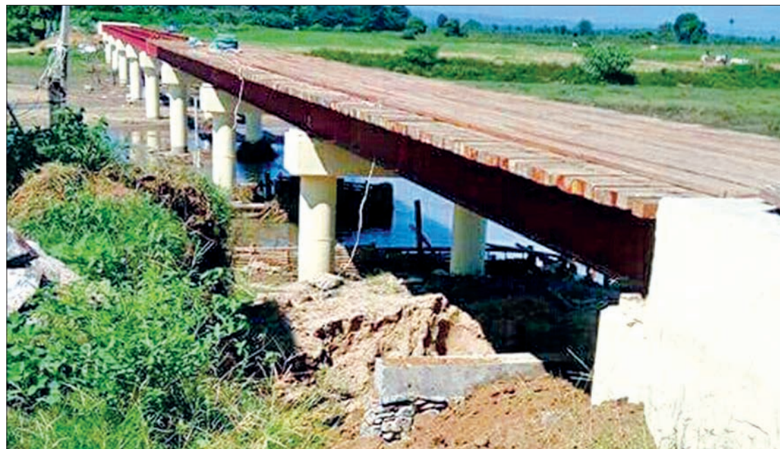
New bridge under construction to link villages of Pobbathiri and Zeyathiri townships. PHOTO: SHWE YE YINT
