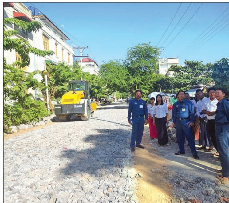
Officials of MCDC inspect progress in construction of road in Chanayethazan Township. PHOTO: THIHA KO KO
