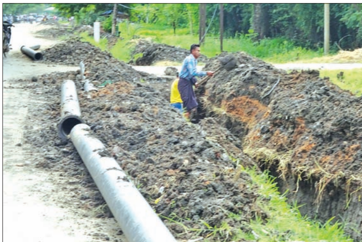
Workers lay a pipeline for water supply service in Mandalay. PHOTO: MAUNG PYI THU
