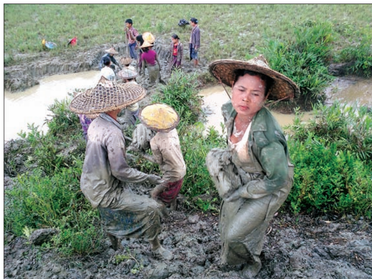
A Tat Lan, cash-for-work labourer from Yoe Sa Nwin village works to repair the village embankment following recent floods in Myanmar.
