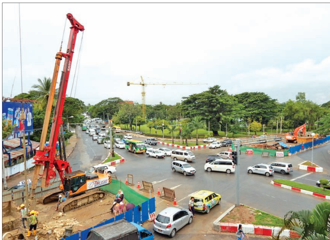
An overpass under construction at Kokkine Junction in Bahan Township. PHOTO: TIN HLA MAUNG
