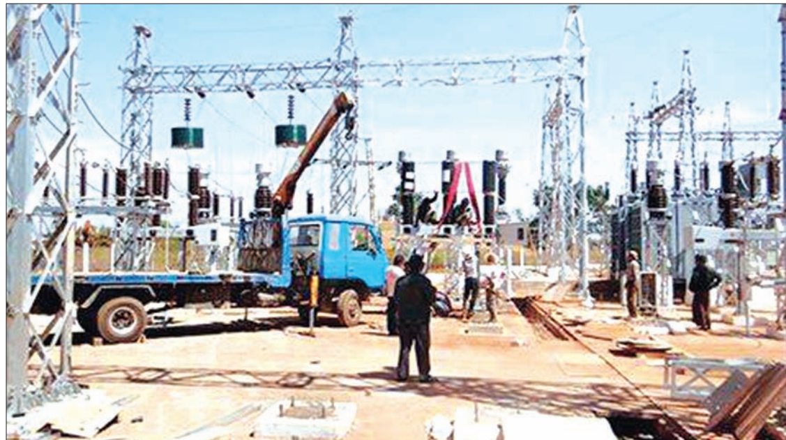
A 66/11 KV 20 MVA sub-station under construction in Inlay Hotel Zone. PHOTO: MAUNG MAUNG THAN
