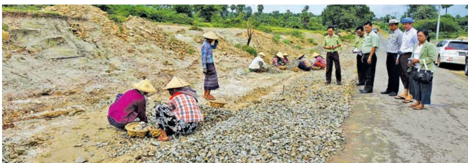
Myohta-Ngazun-Kyauntalone road in Ngazun Township under construction. PHOTO: U ZAW MIN NAING -MYINGYAN
