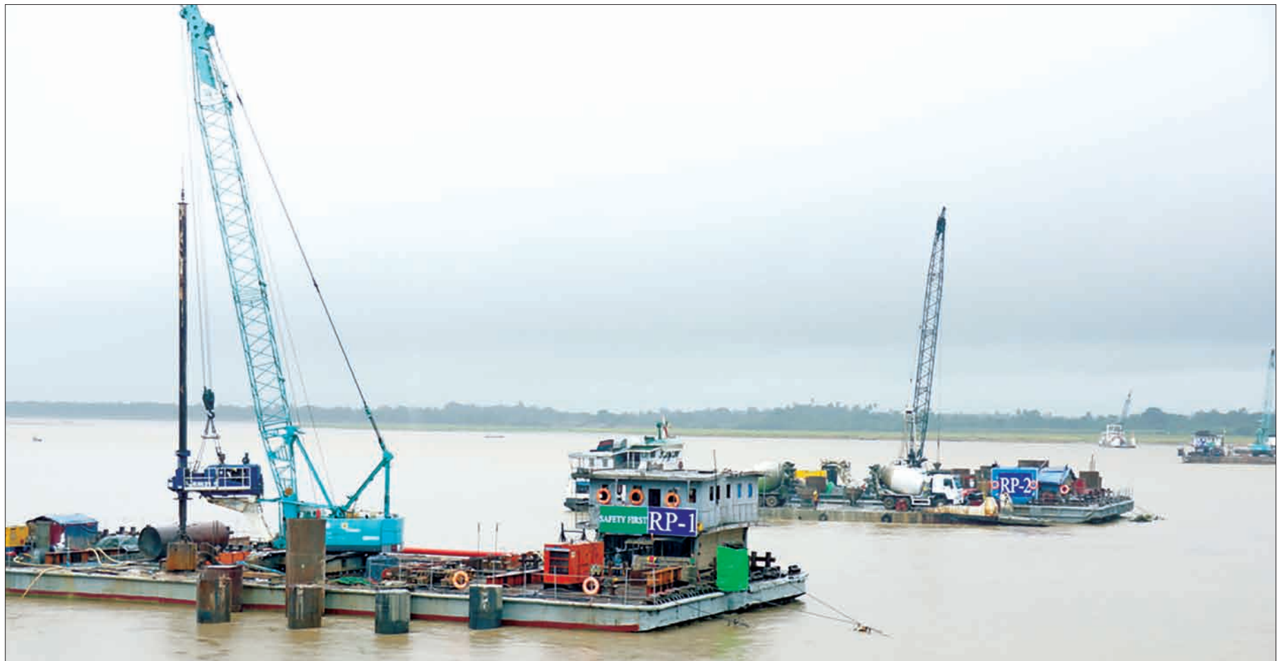
Thanlwin Bridge (Chaungzon) construction project started on 8 February 2015 and expected to complete in December 2016.
