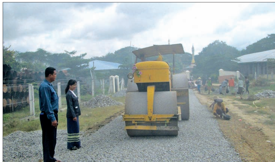
Engineers at work to upgrade a road in Tatkon. PHOTO: TIN SOE LWIN
