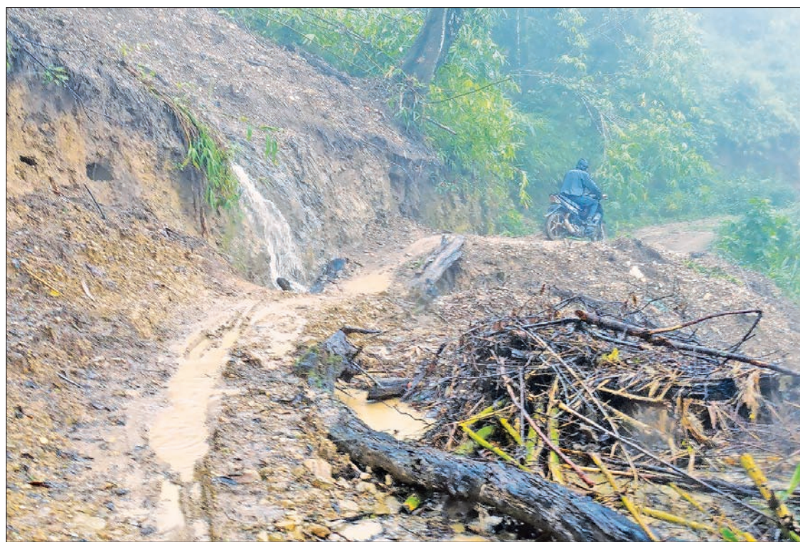
Recent floods in Chin State caused landslides blocking a road leading to a dam in hilly region.—PHOTO: SU HNIN LEH
