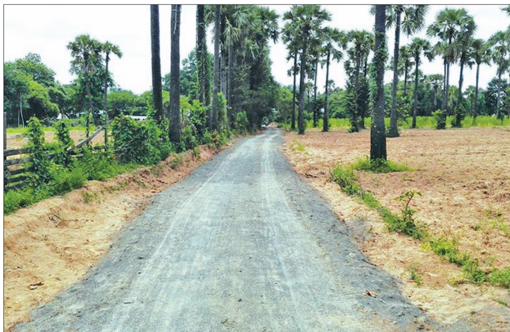
A road linking Thangyigon and Magyisu villages in Kyaukpadaung Township under construction. Ko NAY-KYAUKPADAUNG
