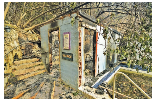
Burned out remains of the popular nudist destination Harbin Hot Springs are seen after the Valley fire roared through the area near Middletown, California on September 14, 2015.—AFP
