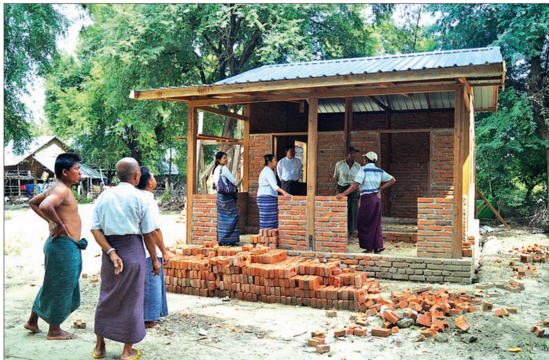
Officials of Information and Public Relations Department from Nay Pyi Taw Council Area inspect progress in construction of rural library in Tatkon Township.—TIN SOE LWIN-IPRD
