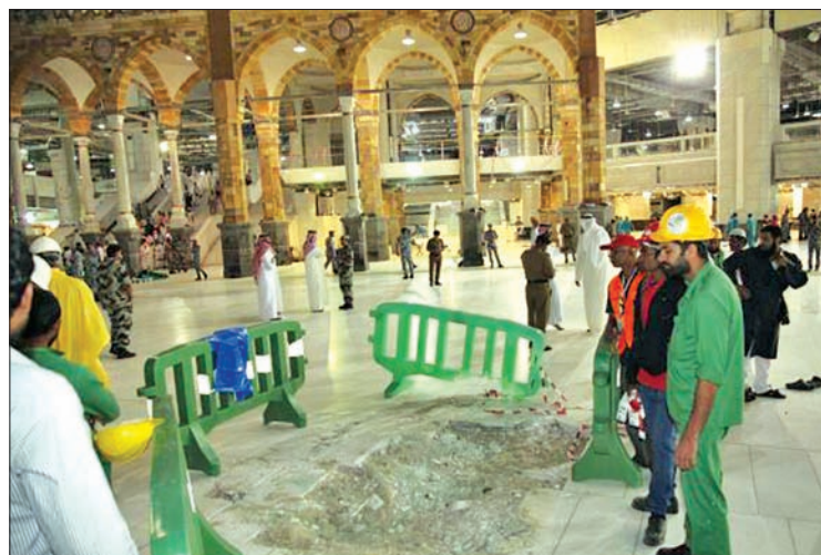
Members of a Saudi emergency crew stand near damage caused by a collapsed crane at the Grand Mosque in the Muslim holy city of Mecca, Saudi Arabia September 11, 2015.—REUTERS
