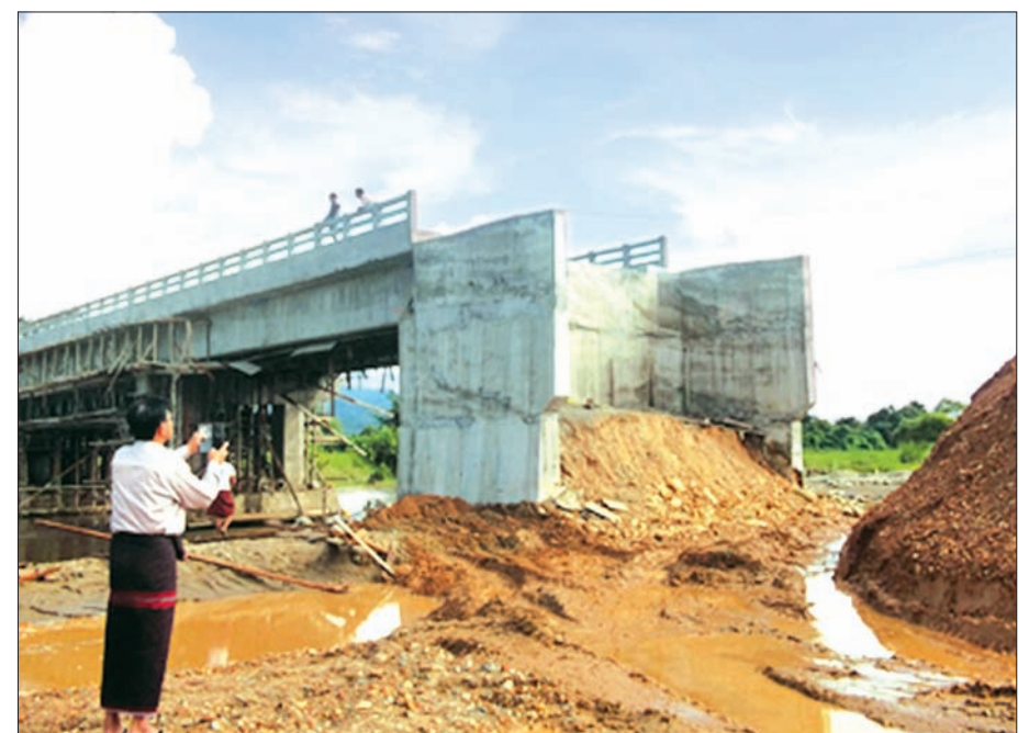
The bridge is expected to complete one year later than its target.—GNLM001
