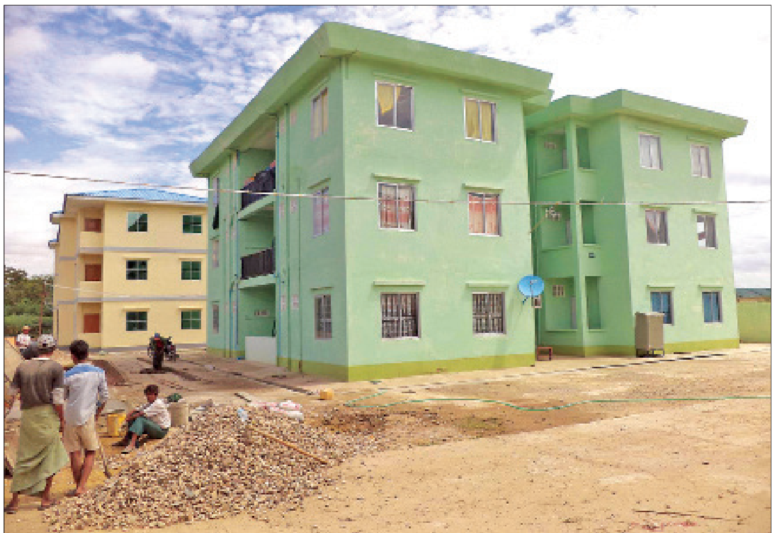
Four apartment buildings for service personnel are under construction with finishing works in Meiktila.—Chan Thar
