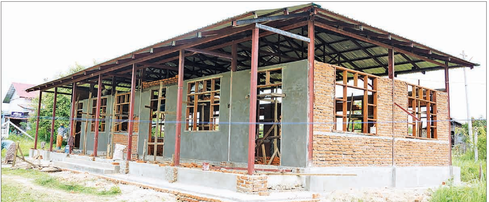
A new school building is under construction at No 97 BEMS (Branch) in Pobbathiri Township.—SHWE YE YINT
