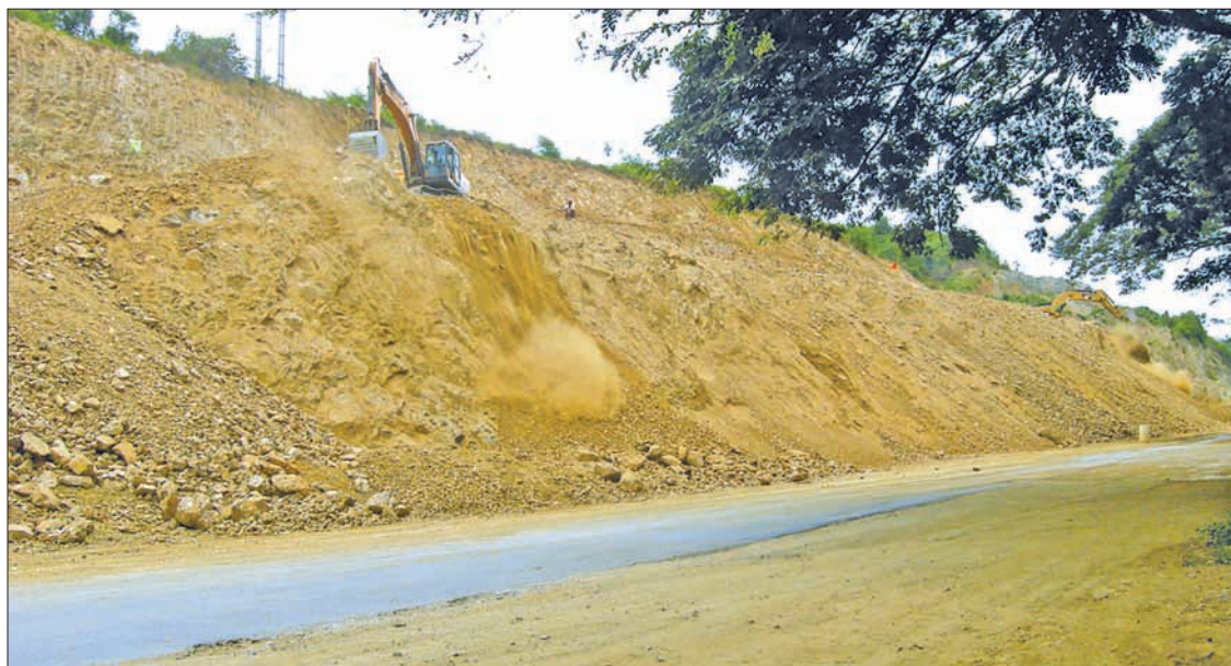
A road section of Yangon-Mandalay Highway being expanded in Tatkon Township.—TIN SOE LWIN
