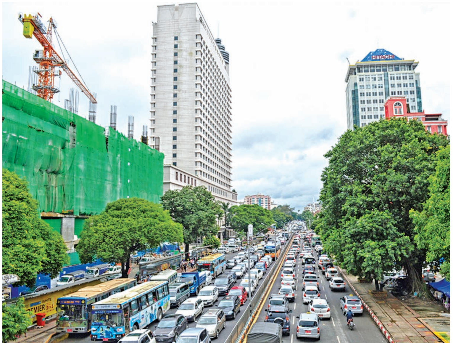
A construction site in the heart of the commercial capital of Yangon. Experts have said that the sluggish state of Myanmar's property market will continue until the year end.— PHOTO: YE MYINT
