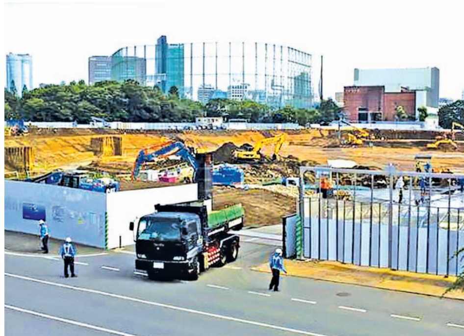
A truck leaves the construction site of Japan's new National Stadium in Tokyo July 17, 2015. —REUTERS
