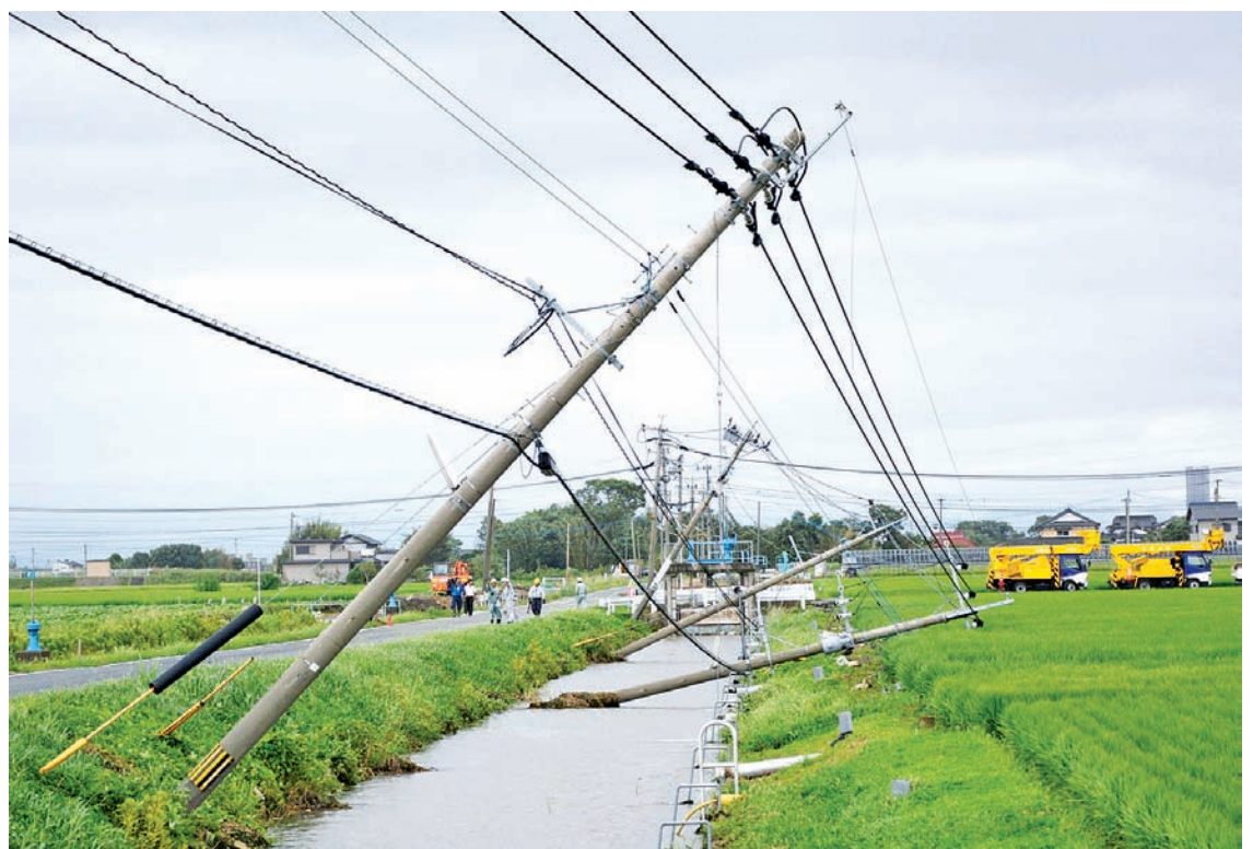
Power poles damaged due to strong winds caused by Typhoon Goni are seen in Kamimine town, Saga Prefecture, Japan, in this photo taken by Kyodo August 25, 2015. Japanese authorities advised 280,000 people to evacuate their homes as a typhoon lashed southern Kyushu island and western Japan on Tuesday, bringing torrential rains and winds gusting over 110 miles an hour (180 kph).—KYODO NEWS
