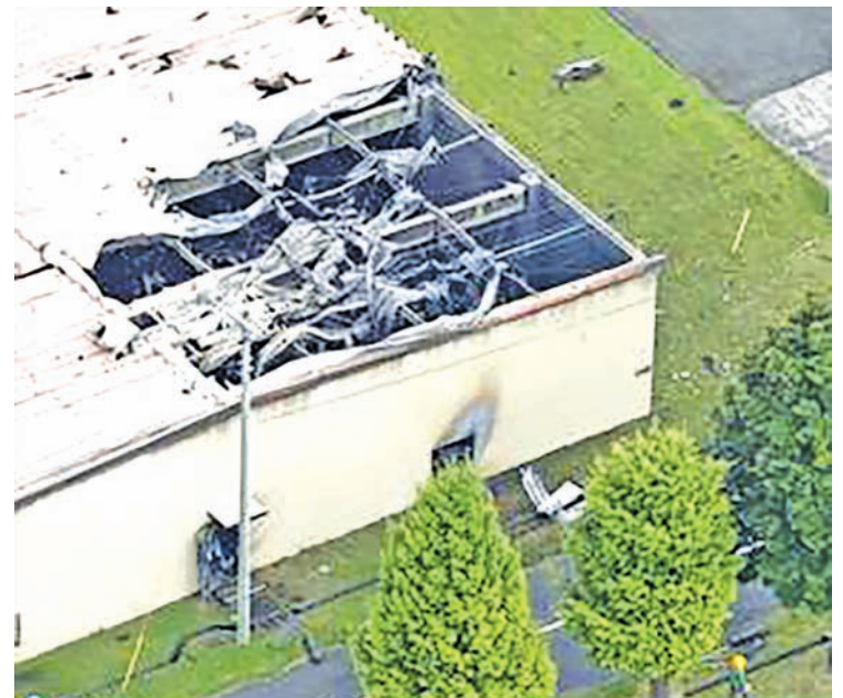
Photo taken Aug. 24, 2015, from a Kyodo News helicopter shows a burnt warehouse at a U.S. military base in Sagami, some 40 kilometers southwest of Tokyo, where an explosion caused the building to burst into flames. Kanagawa prefectural police said the U.S. military will look into the cause of the incident as the fire occurred within the base premises.—KYODO NEWS
