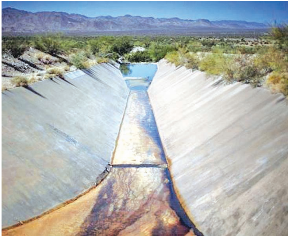
A dry canal is seen running off the Colorado River Aqueduct, in Hayfield Lake, California, United States May 18, 2015.—REUTERS
