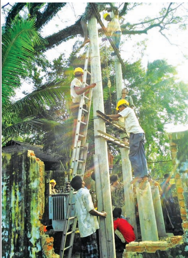
Electric engineer staff fix electrical cables and posts battered by Cyclone Komen in Maungtaw.—IPRD
