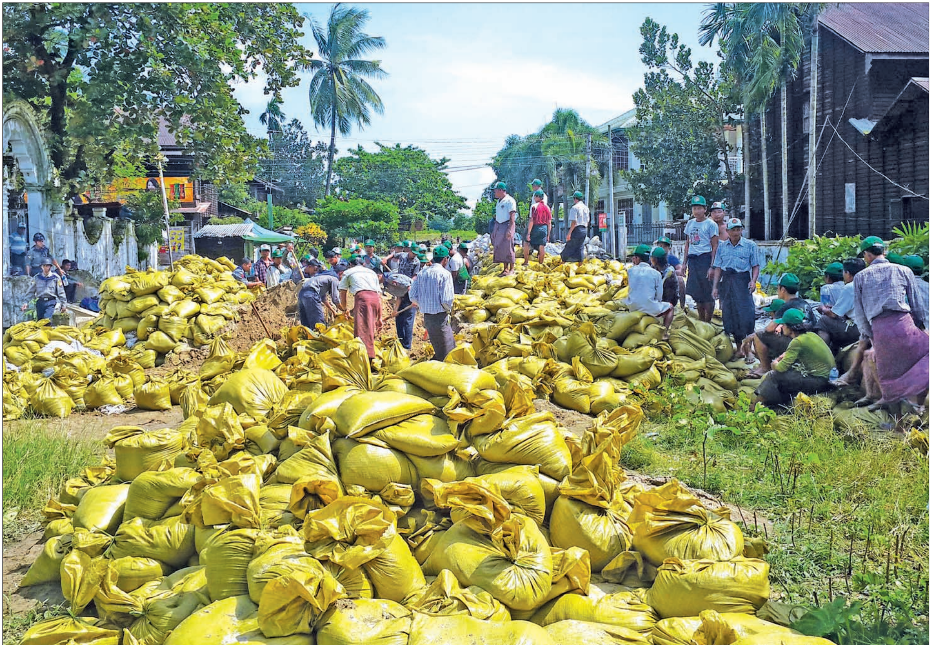
Volunteers lay sandbags on the bank of the Ayeyawady River in Nyaungdon to hold back rising waters. PHOTO : THAPYAY TUN (NYAUNGDON)
