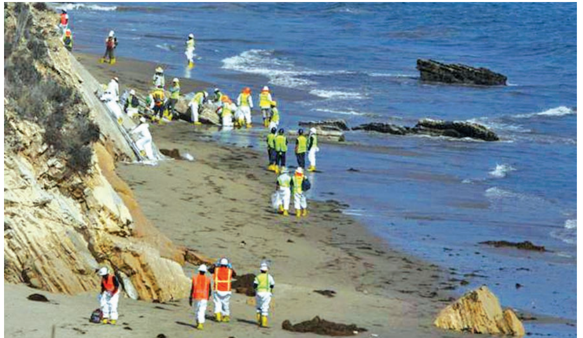
Workers continue to clean the sand and rocks south of Refugio State Beach where an oil spill on May 19, 2015 sent as much as 2,400 barrels of barrels of oil into the Pacific Ocean in Santa Barbara County, California July 30, 2015.—REUTERS
