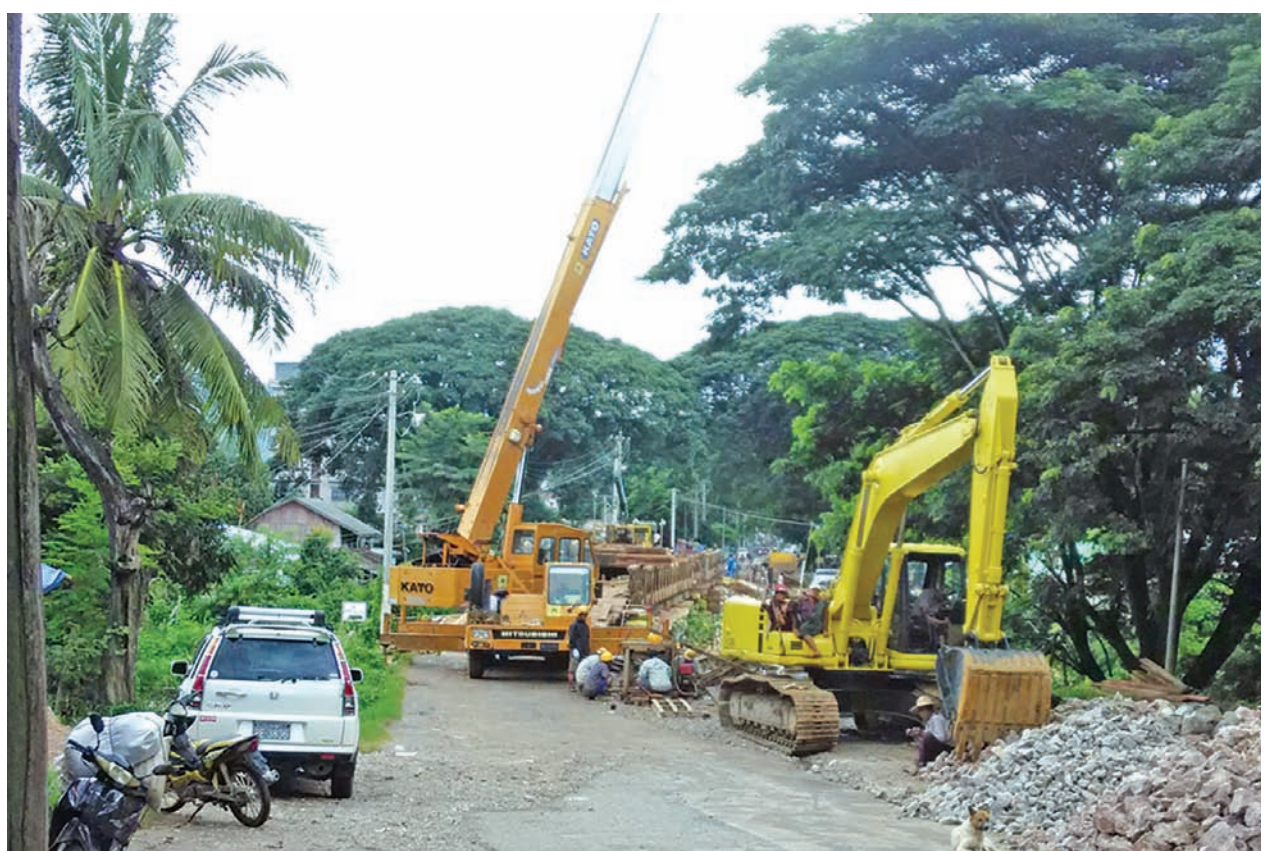
A bailey bridge is under construction across Nampaw Creek in Hsipaw Township, Shan State, with 75 percent complete on 30 July.—SAI TUN THEIN (HSIPAW TOWNSHIP IPRD)
