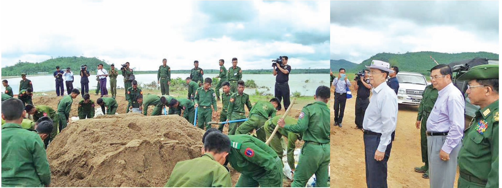
President U Thein Sein and Commander-in-Chief of Defence Services Senior-General Min Aung Hlaing encourage military service personnel volunteering for repairing a dam which was damaged by the flood caused by torrential rain in Sagaing Region recently.—MNA
