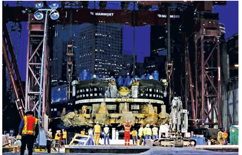
Workers look on as they lift the machine head from Bertha, the world's largest tunnel-boring machine, from an access pit for repairs in Seattle, Washington on 30 March, 2015.—REUTERS
