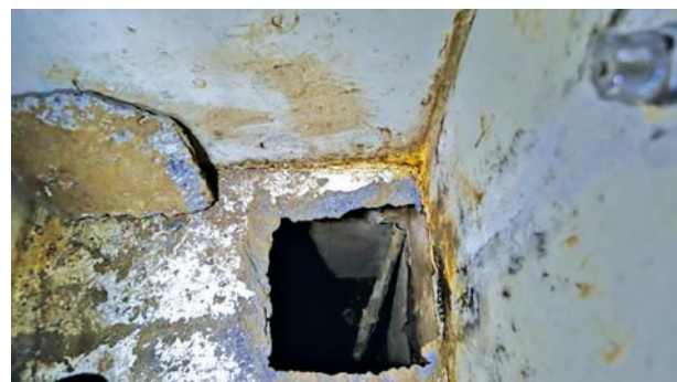
A view of the opening of a tunnel, which is connected to a warehouse, inside drug lord Joaquin ‘El Chapo’ Guzman’s cell in the Altiplano Federal Penitentiary, where he escaped from, in Almoloya de Juarez, on the outskirts of Mexico City, on 15 July, 2015.—REUTERS
