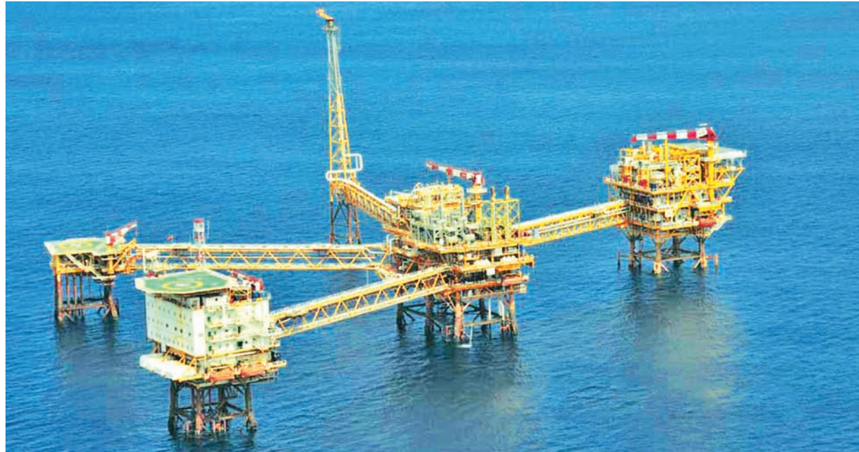
Photo of Yadana gas field located in Andaman Sea, approximately 60 kilometers offshore the nearest landfall in Myanmar. With a huge estimated reserve and international giants awarded onshore and offshore blocks, Myanmar has a huge potential in the oil and gas sector beyond 2015.
