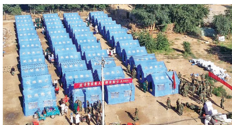
Tents are erected in quake-hit Pixna Township of Pishan County of Hotan Prefecture, northwest China's Xinjiang Uygur Autonomous Region, on 4 July, 2015. A 6.5-magnitude earthquake rocked Pishan County of Hotan Prefecture at 9:07 am (0107GMT), with the epicenter recorded at 37.6 degrees north and 78.2 degrees east, according to the China Earthquake Networks Centre (CENC). Relief materials are being carried to the quake-hit regions.—XINHUA
