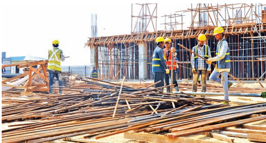
Skilled workers at construction projects in Thilawa Special Economic Zone.—PHOTO: MYAT THANDA
