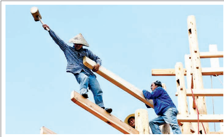
People of the Dong ethnic group take part in the construction of a drum tower at Rentang Village of Sanjiang Dong Autonomous County, southwest China's Guangxi Zhuang Autonomous Region, on 27 June, 2015. Drum tower is a landmark structure of the villages of the Dong ethnic group where important public affairs are dealt with. XINHUA
