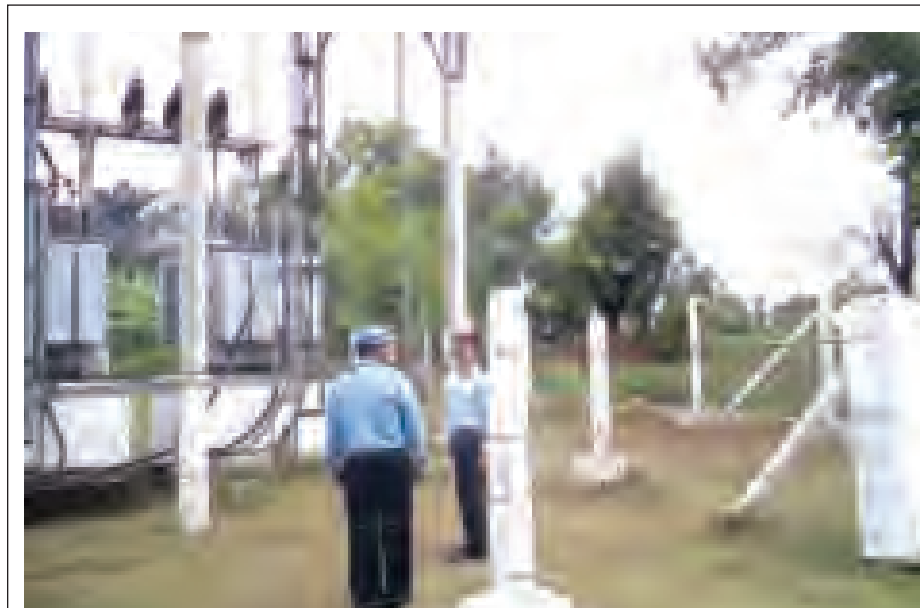
Ayeyawady Region Electrical Engineer U Aung Than inspects 2x1250KVA sub-power station, 33 KV and 11KV power lines in Kyaunggon Township on 11 June.—DAVID (KYAUNGON)
