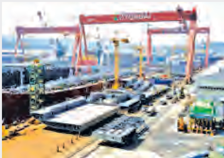
Part of the structure of a ship (bottom C) is transported at Hyundai Heavy Industries' Shipyard in Ulsan, South Korea, on 13 May, 2015.—REUTERS
