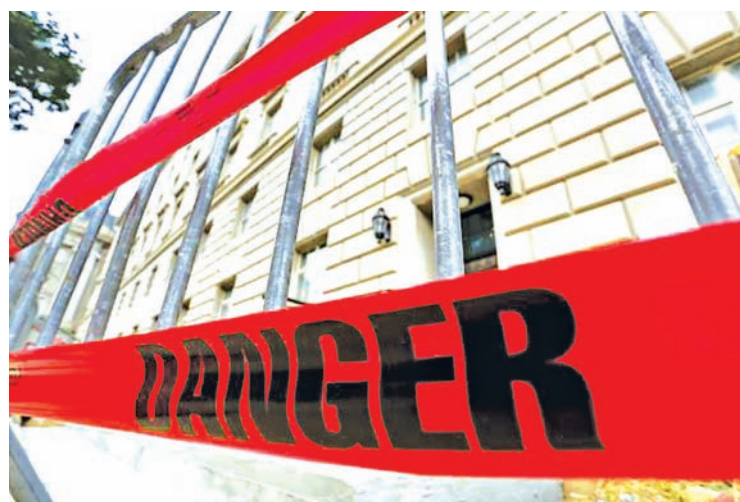
Plastic caution tape marks a small construction area on the exterior of the US Internal Revenue Service (IRS) building in Washington on 27 May, 2015.—REUTERS
