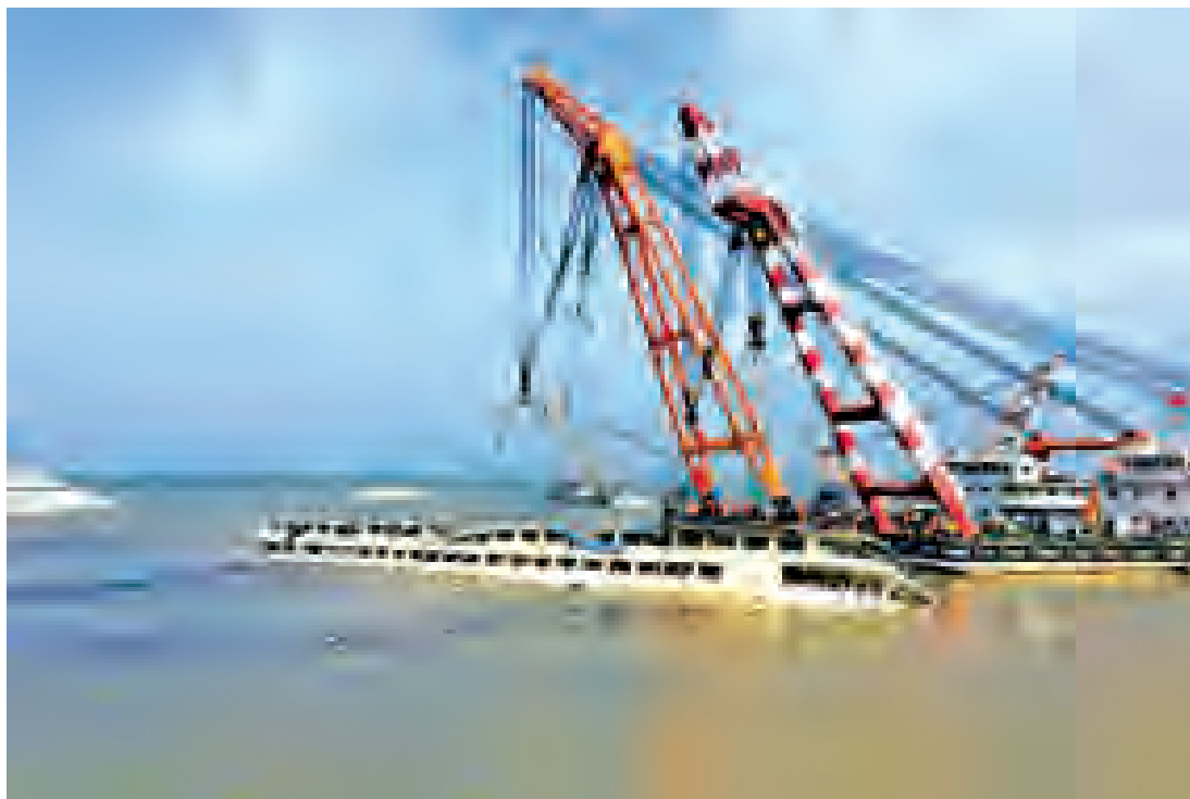
Cranes work on righting the capsized Eastern Star cruise ship at the Jianli section of the Yangtze River, Hubei Province, China, on 5 June, 2015. REUTERS
