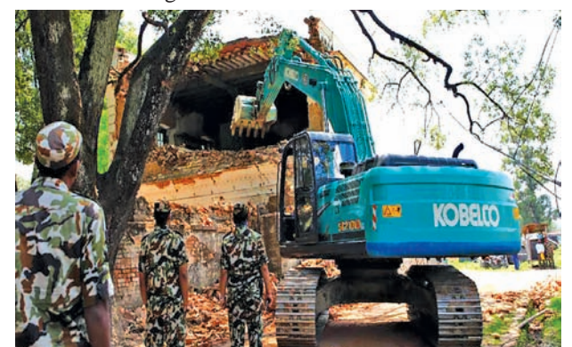
Nepal Army personnel demolish a damaged house in Kathmandu, Nepal, on 23 May, 2015.—XINHUA
