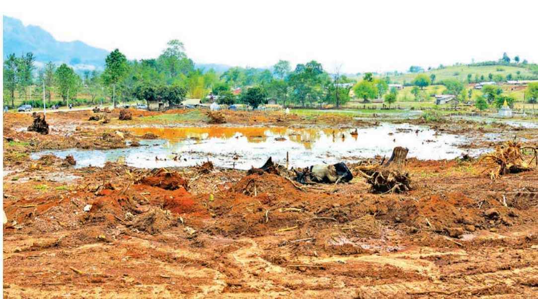
Vice President Dr Sai Mauk Kham views site chosen for construction of fire station near Naungmon Village in Lashio Township.—MNA
