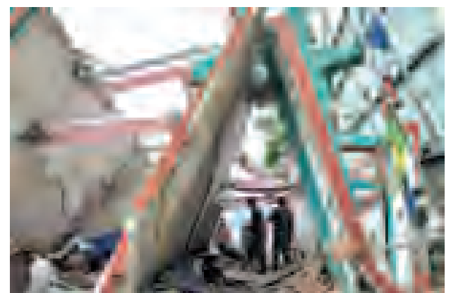
Nepalese military personnel search for bodies inside a collapsed building after Tuesday's earthquake at Charikot village, in Dolakha, Nepal, on 15 May, 2015.
