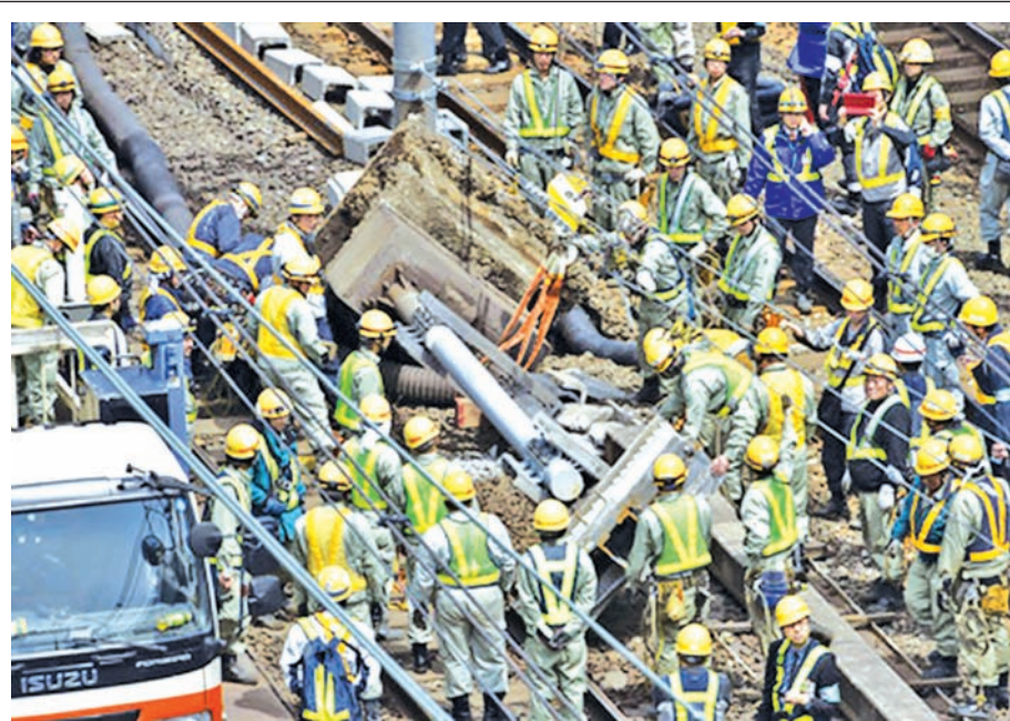
Photo taken on 12 April, 2015, shows collapsed cable-supporting posts on the railway tracks between JR Kanda and Akihabara stations in central Tokyo. The collapse suspended part of the operations of the Yamanote and Keihin-Tohoku lines for more than nine hours.—KYODO NEWS
