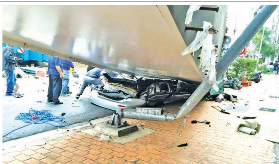
Photo taken on 10 April, 2015 shows the scene of an accident site in Taichung, southeast China's Taiwan. A steel beam fell from a crane at a light rail construction site in central Taiwan's Taichung City on Friday afternoon, killing at least four people and injuring four others, the city government said.—XINHUA
