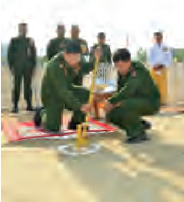
Commander-in-Chief of Defence Services Senior General Min Aung Hlaing drives a stake for construction of a housing estate for war veterans.—MYAWADY
