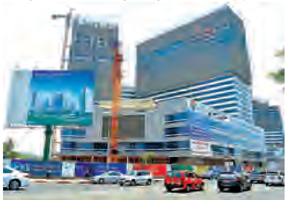
Construction in progress at the worksite of HAGL Myanmar Centre Phase I, for which a soft opening of office buildings and a shopping mall is scheduled for July.— PHOTO: YE MYINT
