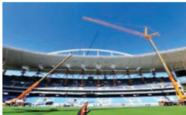
A view of the Joao Havelange Olympic Stadium, undergoing renovation to stage athletic competitions during the Rio 2016 Olympic Games, during the 2nd world press briefing for the games in Rio de Janeiro in this file photo taken on 6 Aug, 2014.—REUTERS
