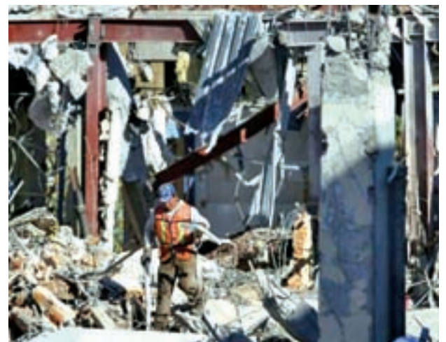
A crew member works to clear debris the day after a deadly gas truck explosion ripped through a maternity hospital in Mexico City, on 30 Jan, 2015.—REUTERS
