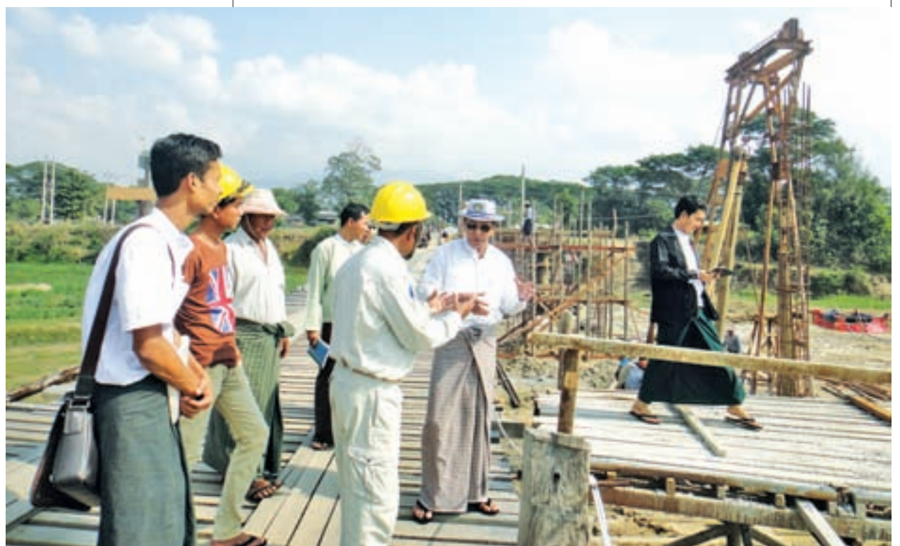
Nay Pyi Taw Council member U Myint Shwe views progress of reinforced concrete bridge crossing Hsinthay Creek in Shwemyo, Tatkon Township.
