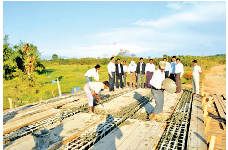
Union Minister U Ohn Myint views construction of concrete bridge on Pamti-Pyihtaung inter-village road.—MNA
