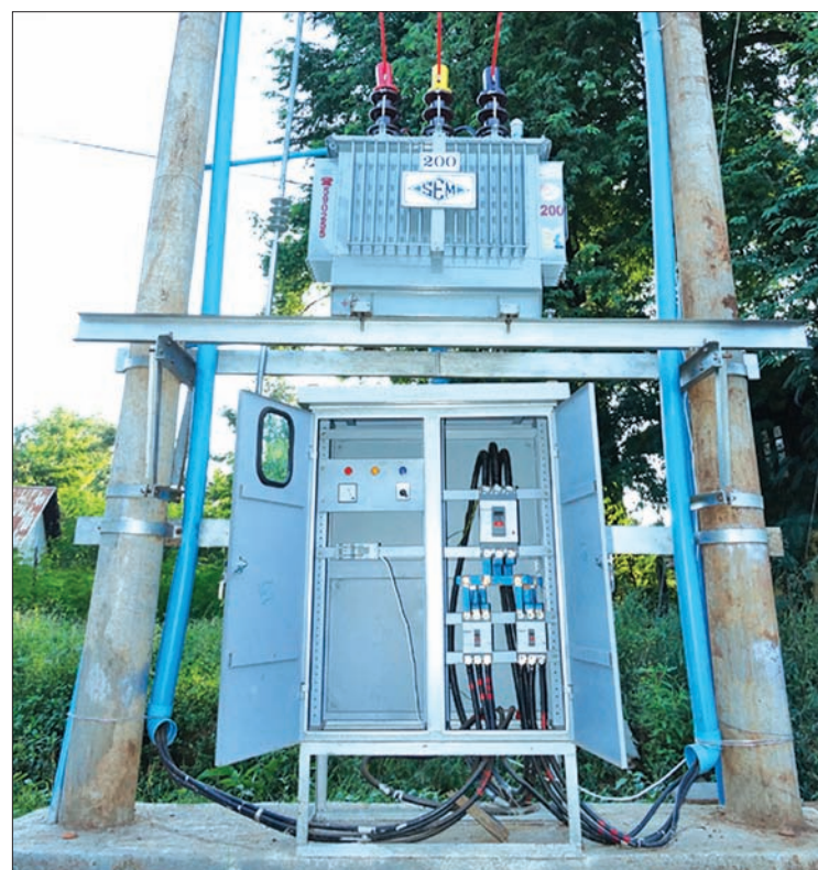
A transformer installed in Linkhe District to supply power to townships in southern Shan State. PHOTO: SAUNG HNIN LATT-IPRD
