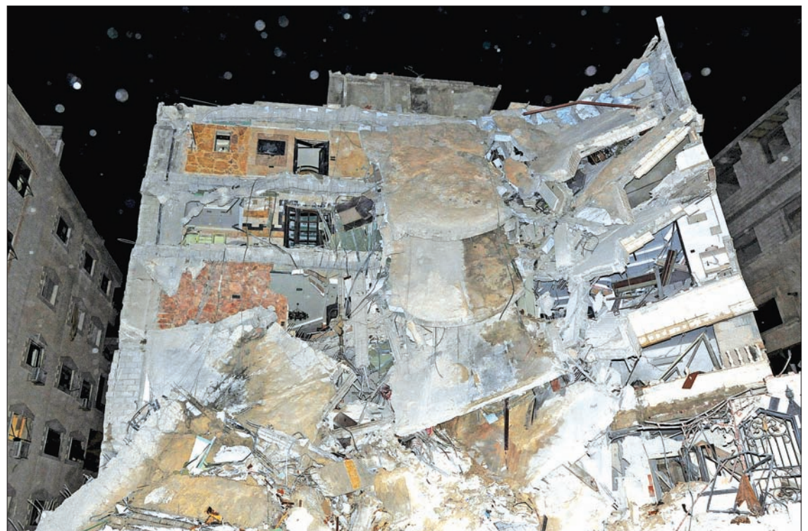
A general view shows a damaged building that was hit by an Israeli strike, killing a Lebanese militant leader Samir Qantar, in the Damascus district of Jaramana, Syria in this handout picture provided by SANA on 20 December. PHOTO: REUTERS
